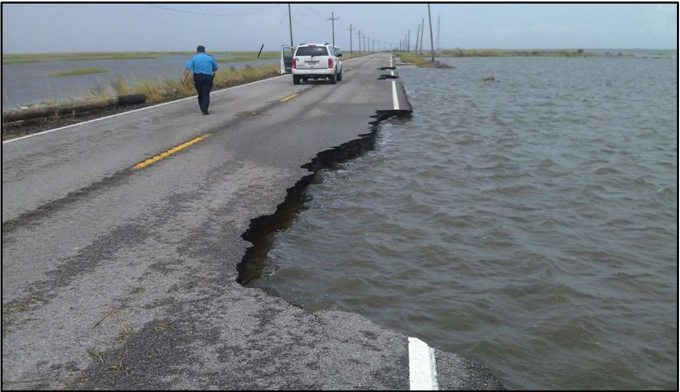
Figure 16. Category 1 Hurricane Isaac brought unprecedented damage to LA 1
