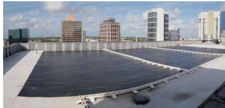
View of the solar roof array on the Higher Education Complex building
