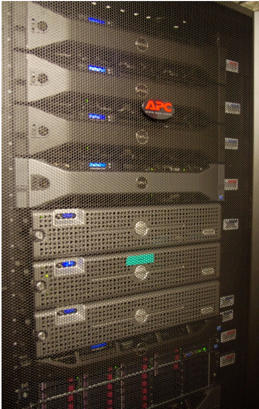
FAU Jupiter Campus Server Room
