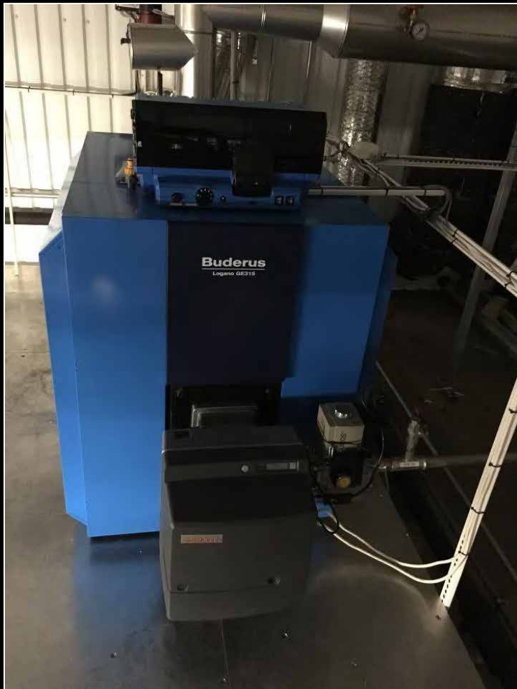
Methane driven boilers
