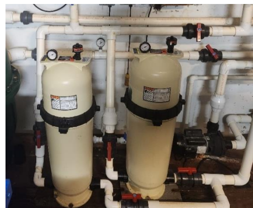
Figure 18. Photograph of modification of cartridge filter plumbing showing parallel flow rather than serial flow as depicted in Figure 16.
