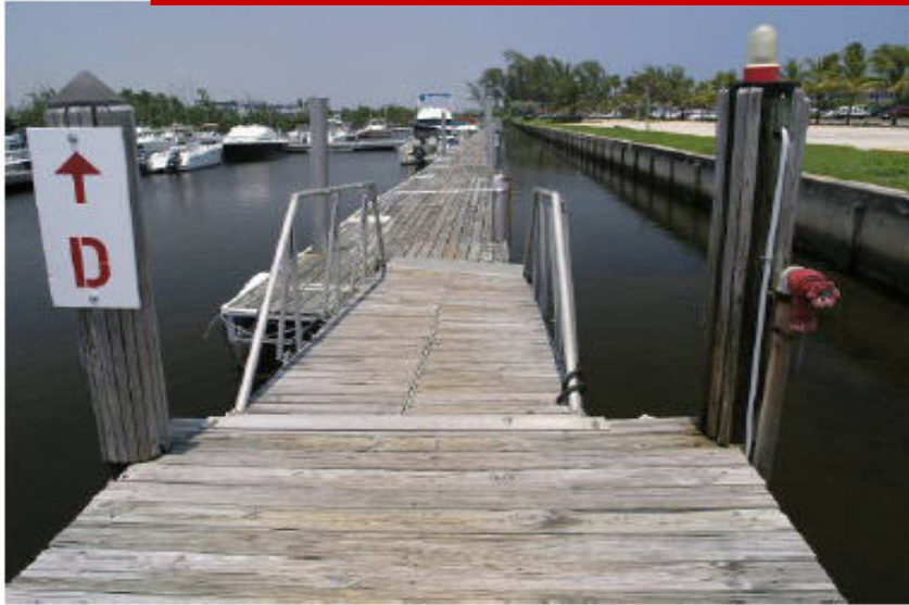
5. View of misaligned ramp from fixed dock to floating
