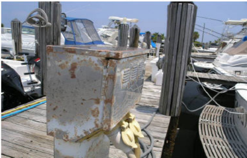
11. View of Power Pedestal
