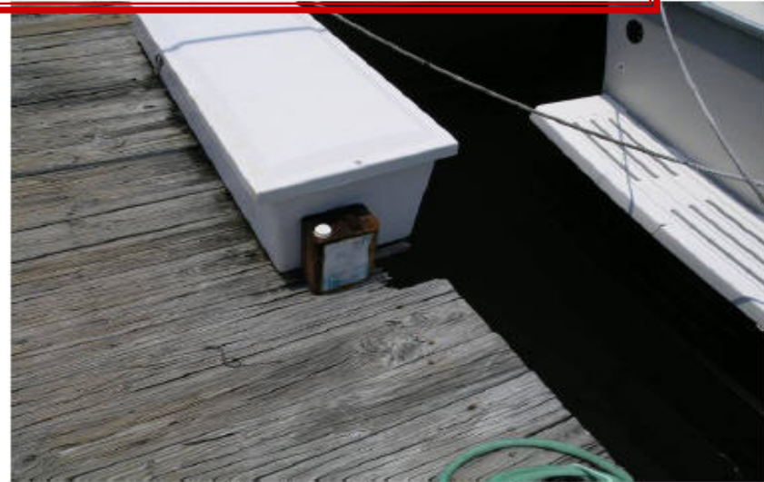
10. View showing broken decking
