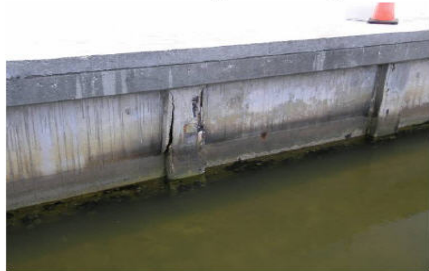
12. View of spalling concrete
